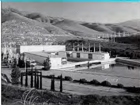
Edmonston Pumping Plant lifts water higher than any single-lift pumping plant in the world – almost 2,000 feet.
