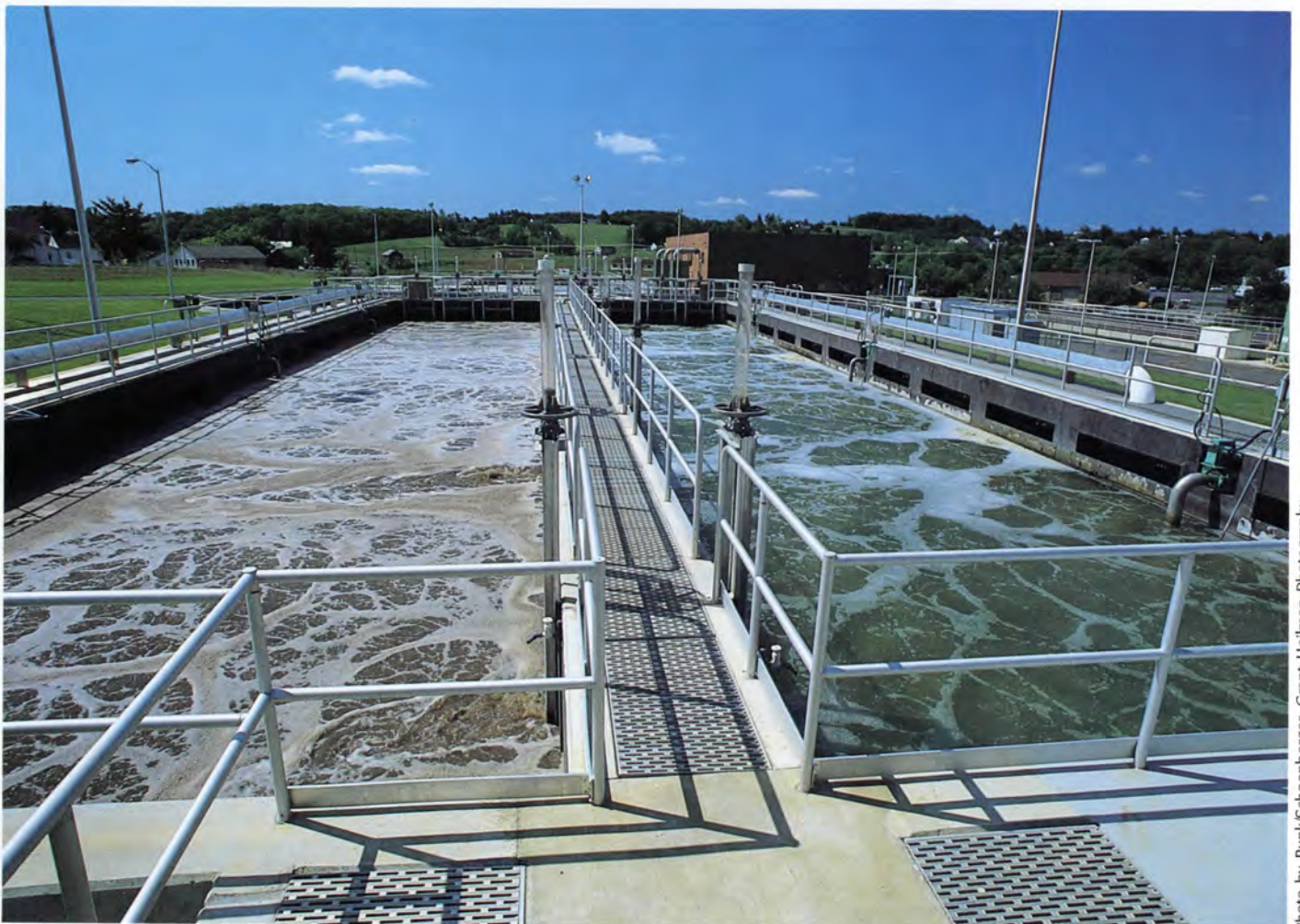
Any wastewater treatment system is attempting to mimic nature — to do what nature does, but to do it more efficiently. Regardless of the water source, public health depends on effective, failsafe treatment processes.
