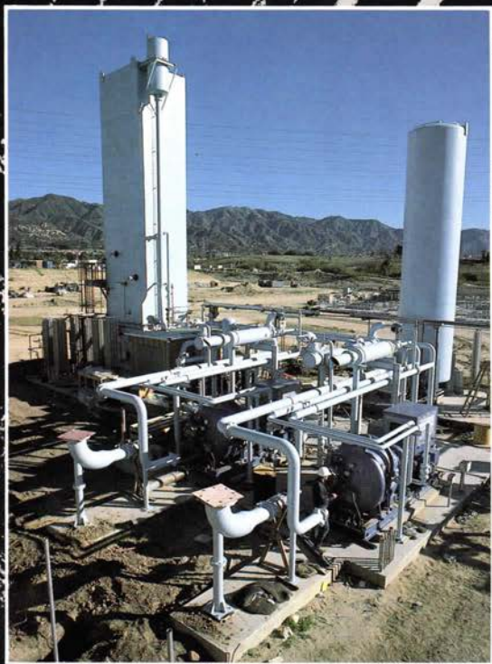
Facility produces pure oxygen for conversion into ozone.
