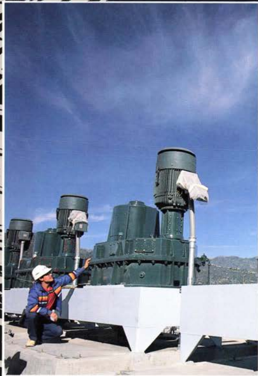
Rapid mix motors are important in the turbidity removal process.
