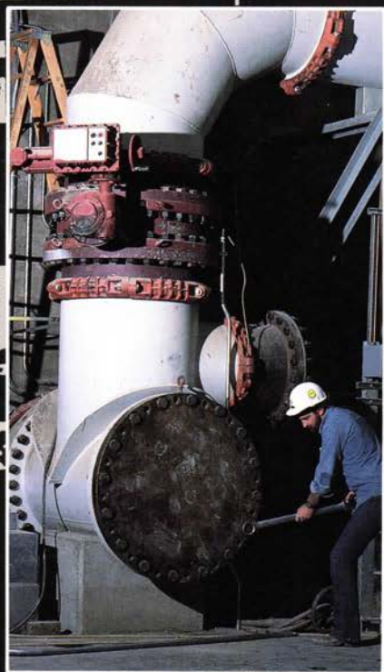
Large pipes route the water to the filter beds.
