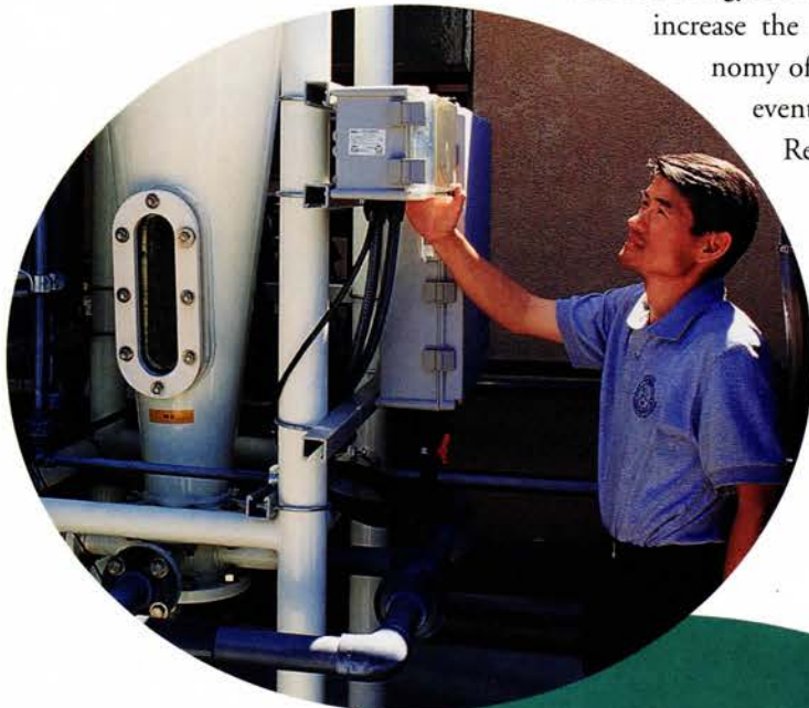
The pilot-scale sulfur-based denitrification plant in Garden Grove tests the feasibility of using specially developed bacteria to "eat" nitrates from groundwater before sending the water to businesses and residences.
