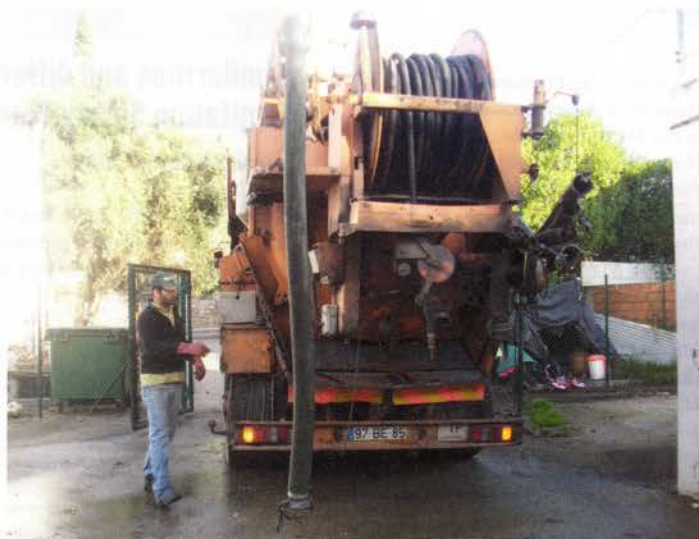
Cleaning of a wastewater pumping station in the Sanitation Safety Plan pilot area in Benavente, north-east of the Portuguese capital Lisbon. Picture courtesy of Acquawise Consulting
