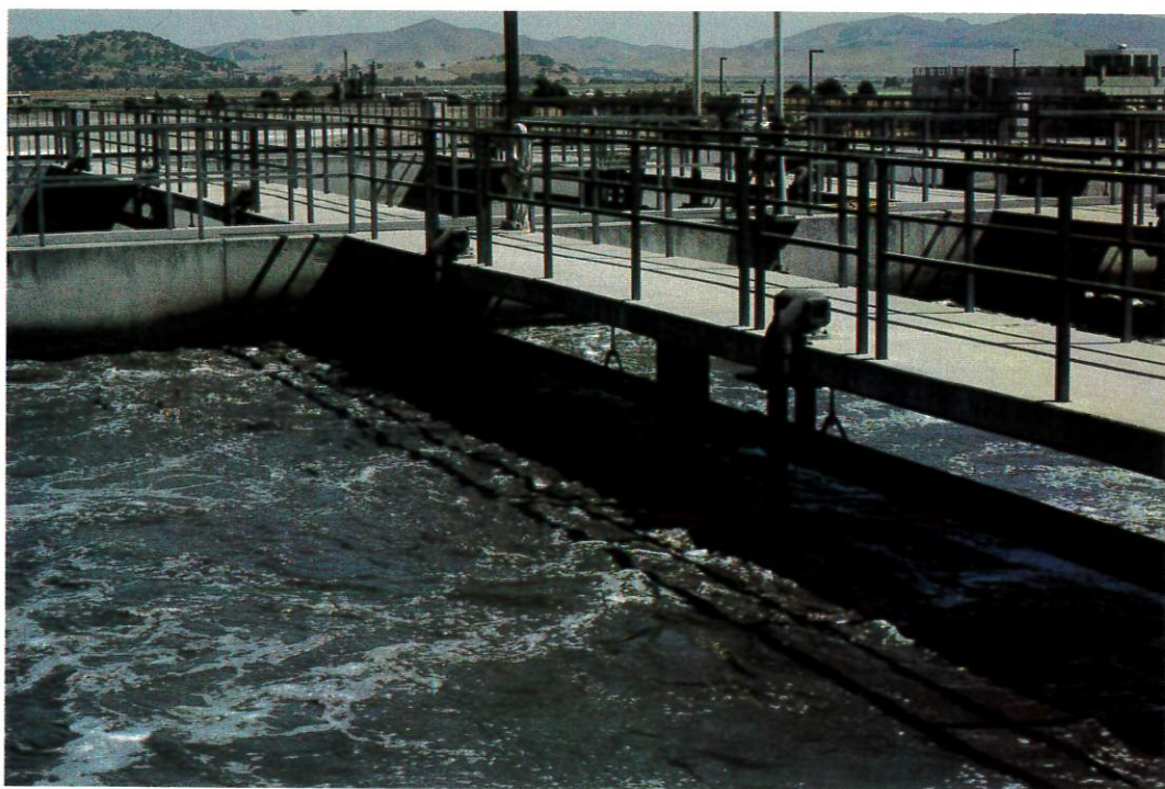
Activated sludge, secondary treatment of municipal wastewater.
