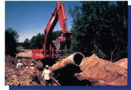
Large-diameter transmission main
