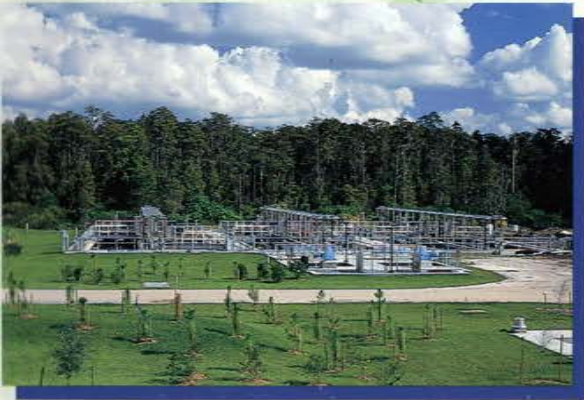
Filtration facility for virus removal
