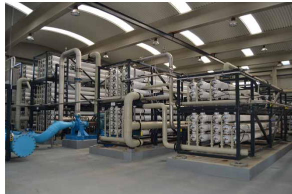
Figure 3 | General view of one of the two-pass RO processes at the Camp de Tarragona AWRP.
